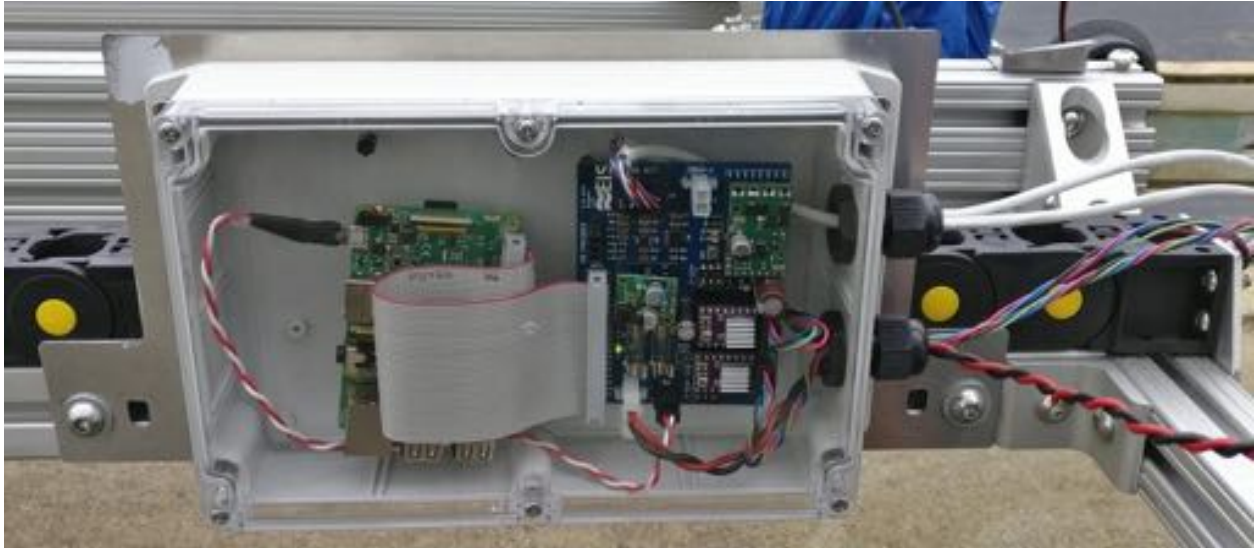
Figure 18: Waterproof electrical enclosure with PCB and RPi inside
